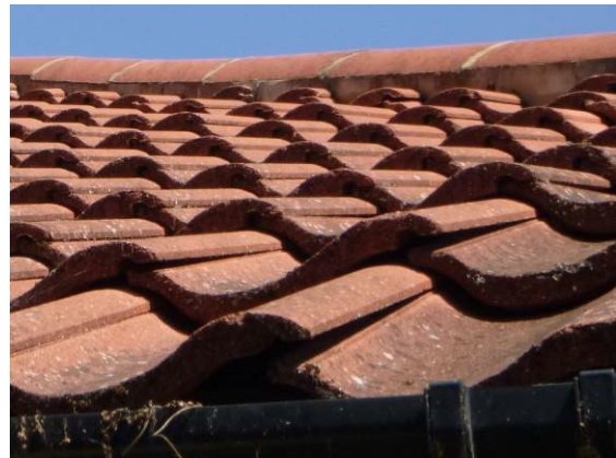
Photograph 4. Small superficial gap underneath pantile (western elevation).
