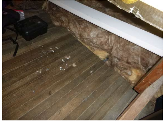
Photograph 14. Partially boarded floor near hatch.
