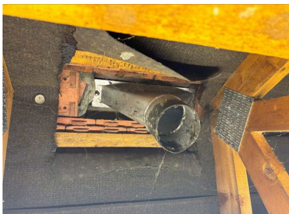
Photograph 11. Gap in felt around a ventilation pipe.
