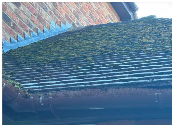
Photograph 5. Roof tiles moss covered on the single storey side extension.
