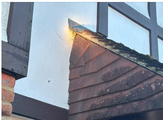
Photograph 10. Gaps around edges of hanging tiles on the porch.
