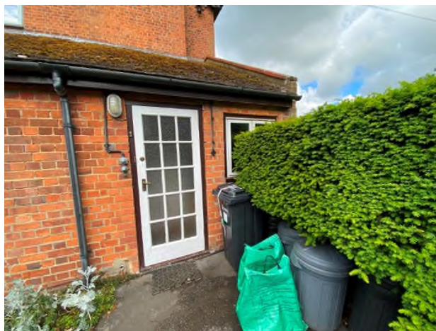
Figure 23: Later and altered window and door openings on the east elevation of the lean-to
