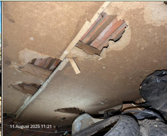
Figure 7: Holes in fibre board in loft void
