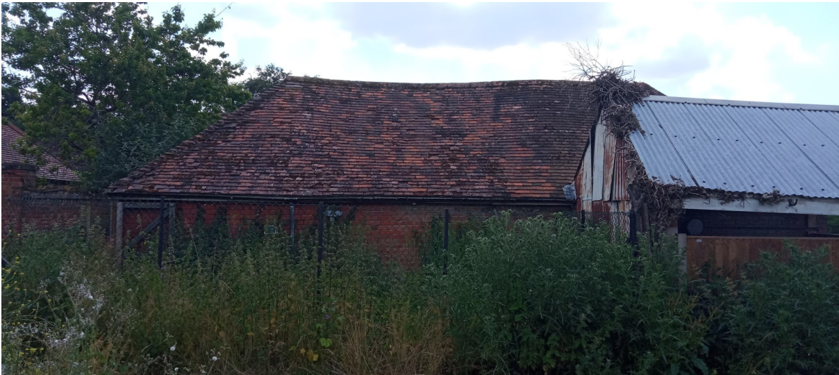
B) Rear elevation of store building showing distortion of main roof ridge
