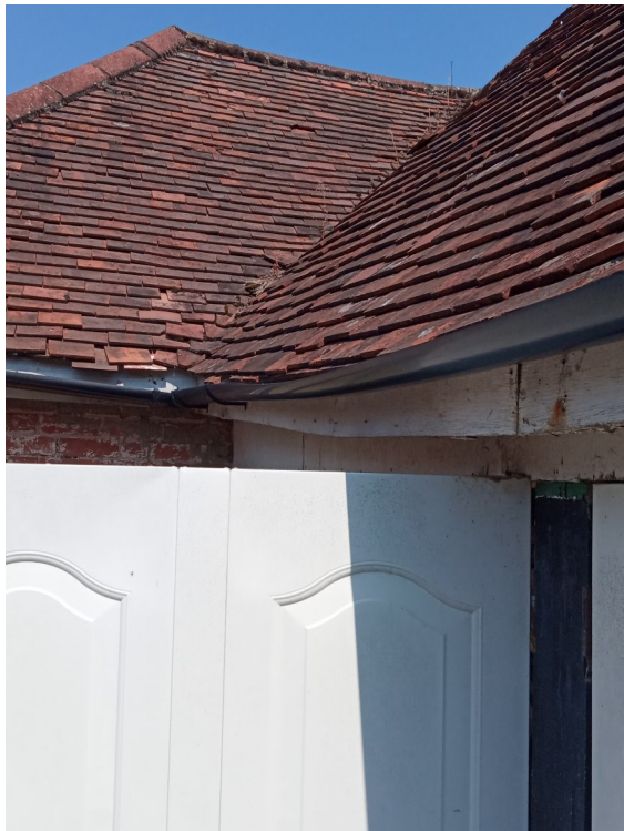
G) Roof deformation at eaves over garage doors
