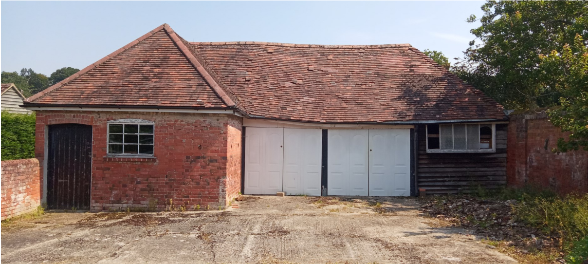
A) Front elevation of store building showing roof deflection over garage doors and affect on main roof ridge and structure
