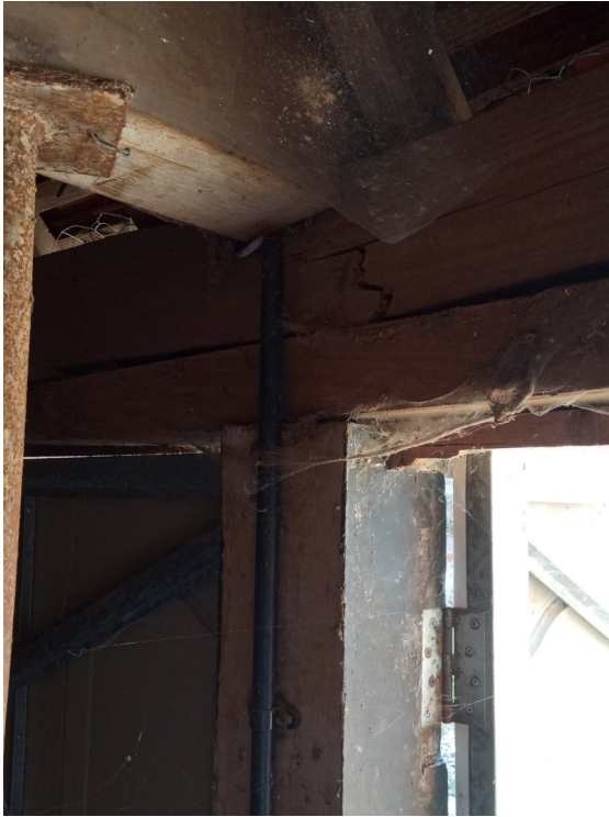
D) Junction of top of post and beam showing deflection and splitting
