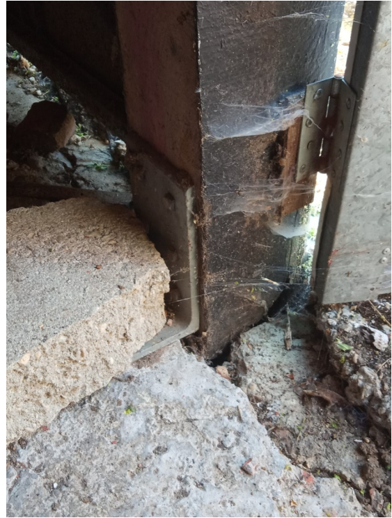
E) Rotten base of existing timber post
