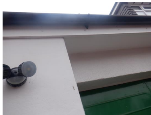
Photograph 10. Tight soffit to painted render wall (northern elevation).
