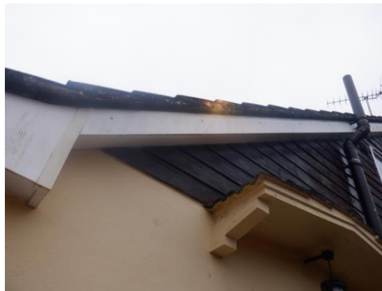
Photograph 8. Superficially crumbling verge mortar (eastern elevation).
