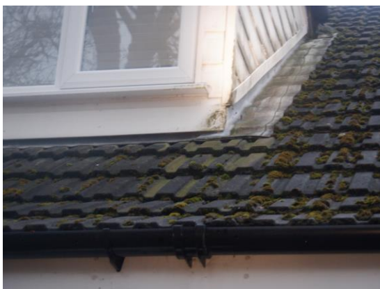
Photograph 5. Slightly lifted lead flashing (northern elevation).
