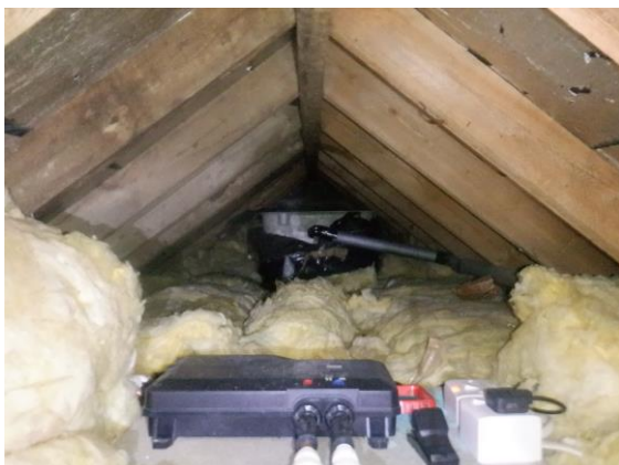
Photograph 11. Fibreglass insulation present throughout (roof void).
