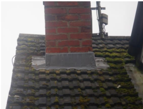
Photograph 7. Slightly lifted lead flashing (northern elevation).
