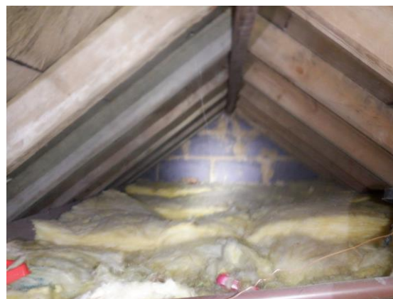
Photograph 14. Cobwebbed along ridge and up to blockwork party wall (roof void).
