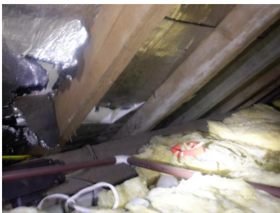
Photograph 13. Tears in foil-backed bituminous roofing felt (roof void).
