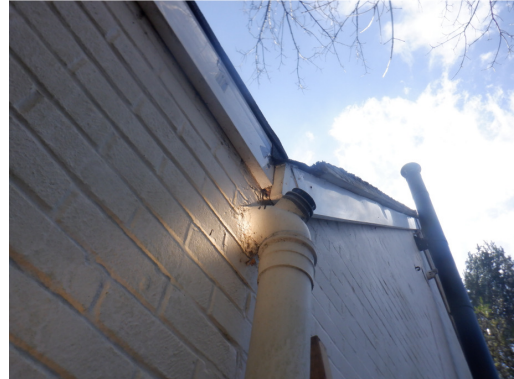
Photograph 7. Small hole in fascia but was backed by timber (western elevation)
