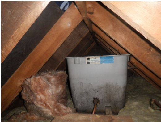
Photograph 11. Cobwebs around water tank.
