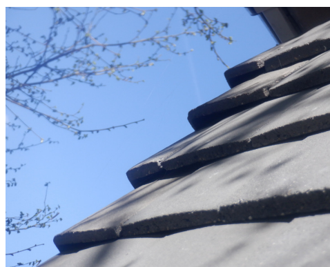
Photograph 5. Gaps in the corner hanging tiles on dormers
