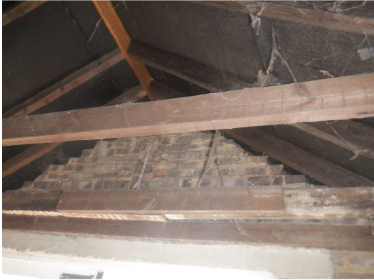
Photograph 12. Heavily cobwebbed garage roof
