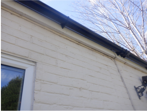
Photograph 6. Barge boards tight to the brickwork (rear elevation)
