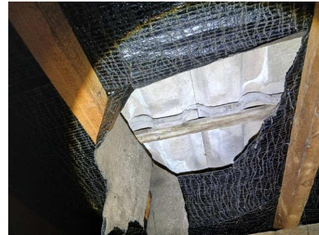
Tears in the internal lining.
