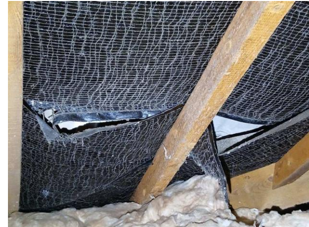
Tears in the internal lining.
