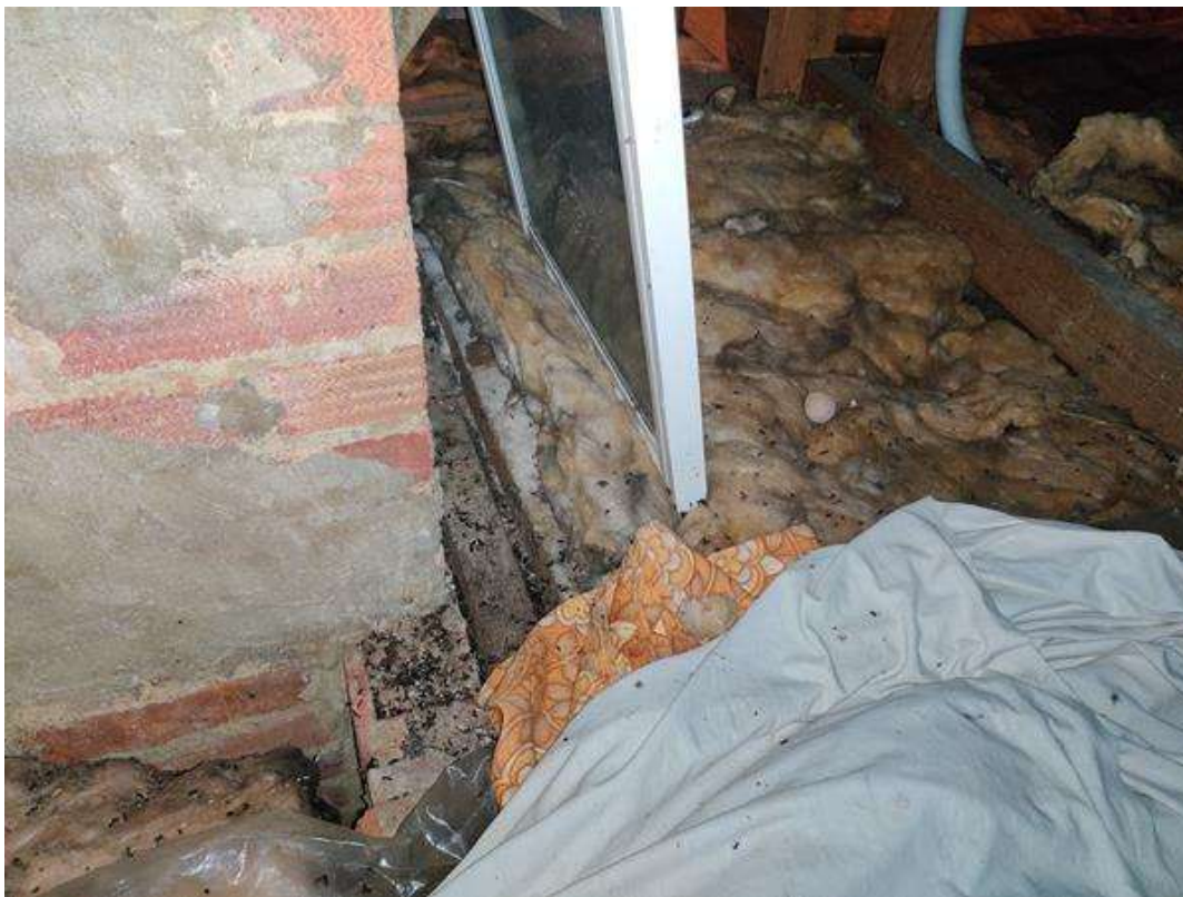
Photograph 4: Bat droppings within the loft beneath the above access point.
