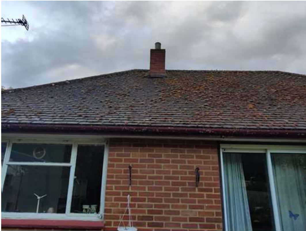
Photograph 3: Gap beneath chimney believed to be used as BLE access point.
