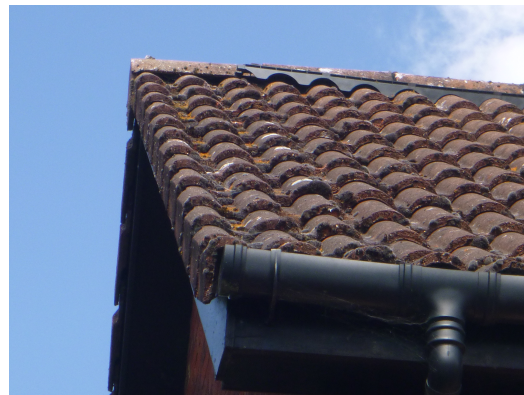
Photograph 4. Broken plastic guard below end ridge tile (front elevation).
