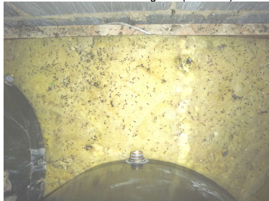
Photograph 19. Accumulation of small bat droppings at base of southern gable (roof void).
