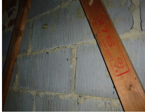
Photograph 17. Small bat droppings stuck to blockwork and timbers on the southern gable (roof void).
