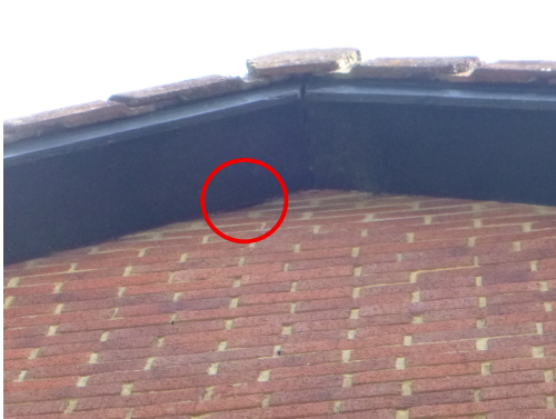
Photograph 7. Gap under soffit near apex of the gable (southern elevation).
