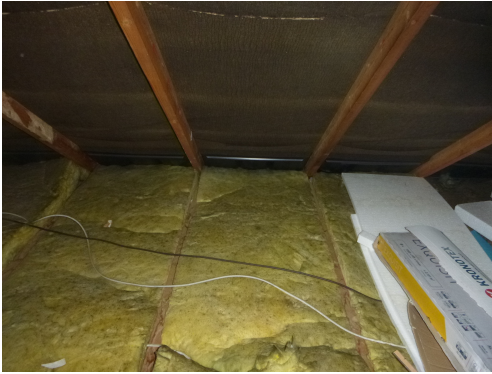
Photograph 11. Fibreglass insulation up to eaves blocked by a plastic guard (roof void).
