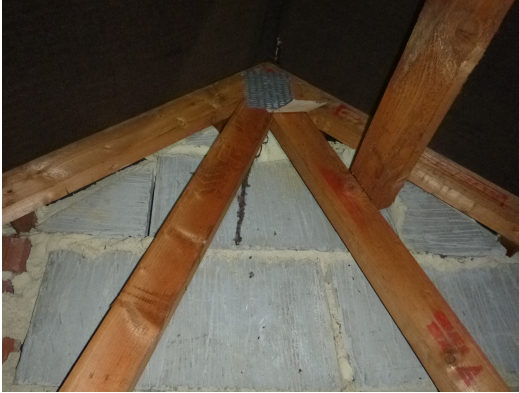
Photograph 16. Gaps above blockwork on the southern gable (roof void).
