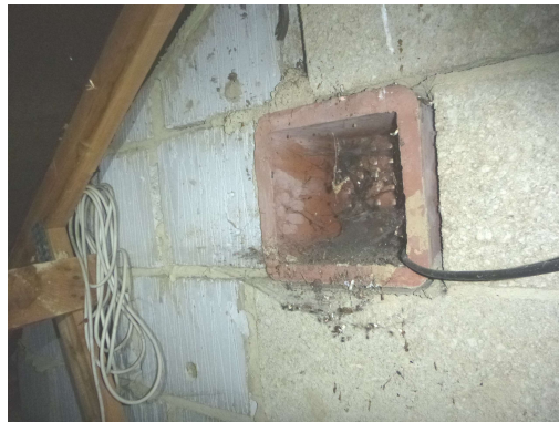
Photograph 14. Cobwebbed vent brick in northern blockwork gable (roof void).
