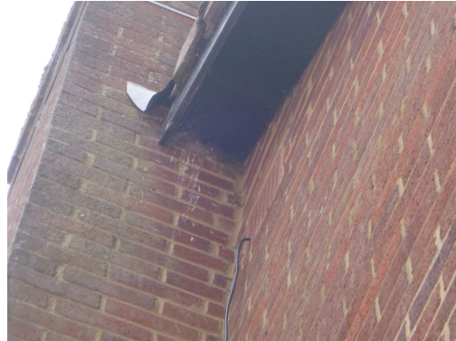
Photograph 8. Lifted lead flashing around chimney and evidence of nesting birds at the soffit (northern elevation).
