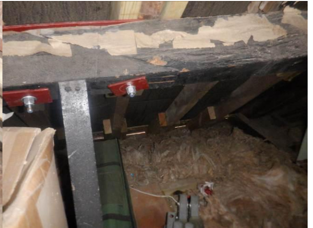
Photograph 17. Daylight visible at eaves
