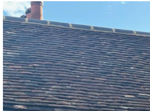
Photograph 4. Raised roof tiles along the front elevation (northwestern view).
