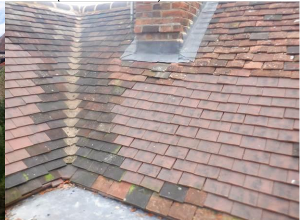
Photograph 6. Uneven roof tiles along the valley (centre of the roof)
