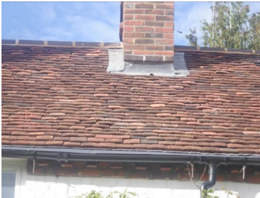
Photograph 3. Raised roof tiles at the rear (southeastern rear view)
