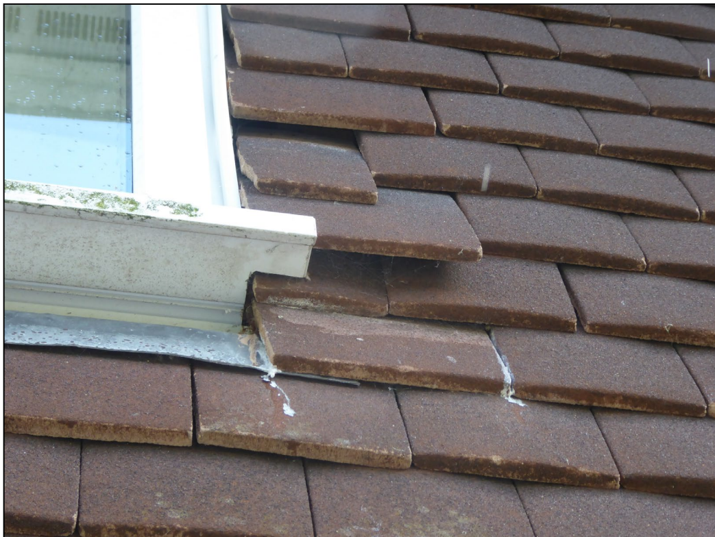
Figure 8. Gaps in hanging tiles on rear elevation. 21 Langhams Way, Wargrave. 20.08.24
