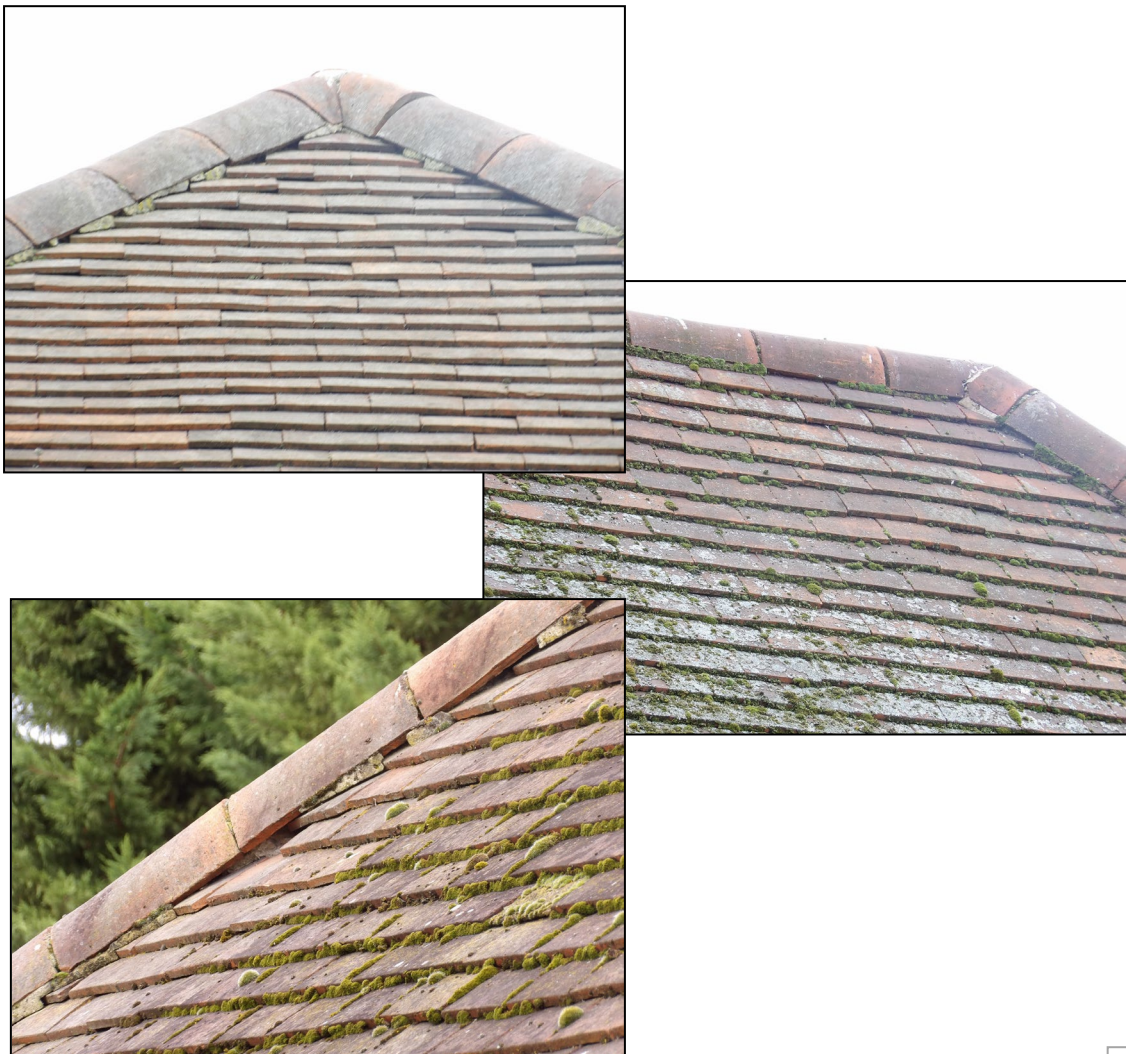
Figure 6. Examples missing mortar from ridge and hip tiles. Blackmoor, Three Mile Cross. 02.09.25
