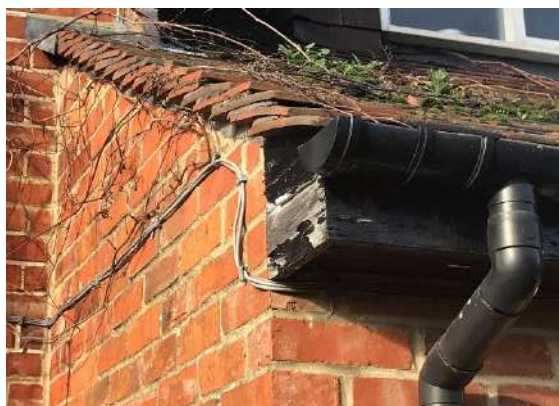
Photograph 11: Lifted tile on the sloped roof porch of No. 83.
