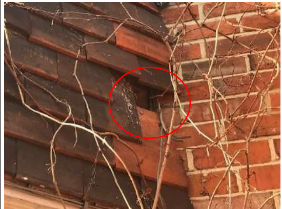
Photograph 12: Missing tile above the bay window on the front elevation of No.83.
