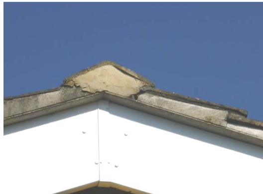
Photograph 6. Slight crack in mortar at gable apex, inspected and deemed too small for bat access.
