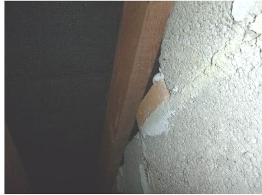
Photograph 18. Gaps around roof timber joints.
