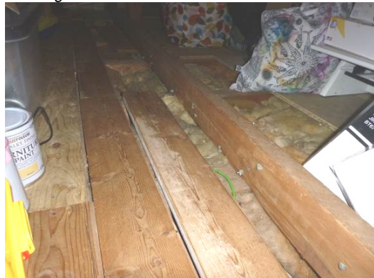
Photograph 16. Fibreglass insulation on floor, boarded in places.
