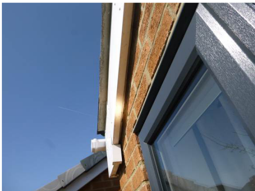
Photograph 7. Gap behind fascia on western side of front gable (Target note 1).
