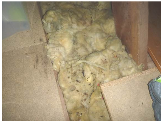
Photograph 14. Rodent droppings scattered on top of fibreglass insulation.
