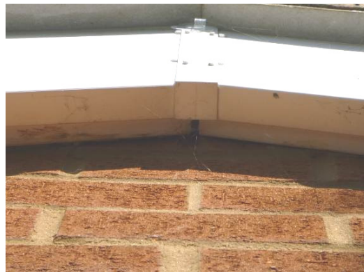
Photograph 8. Small gap at eastern gable apex or converted garage (Target note 3).
