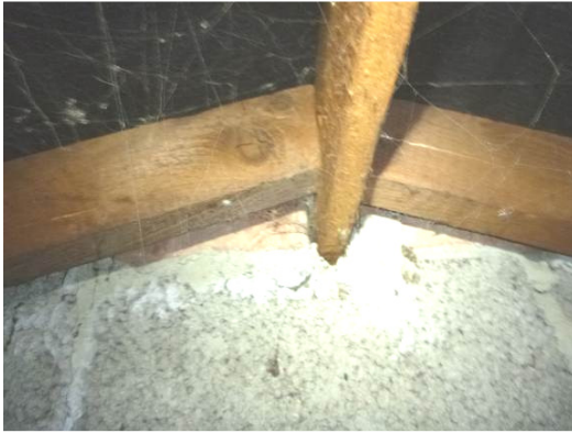
Photograph 17. Small gaps at blockwork apex.
