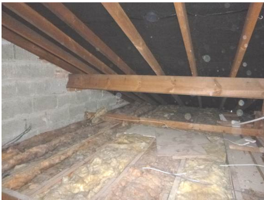
Photograph 13. Fibreglass insulation on floor, boarded in places.
