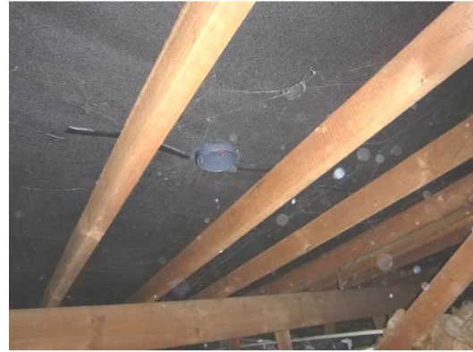
Photograph 12. Bitumen reinforced roof liner with occasional gaps and tears.
