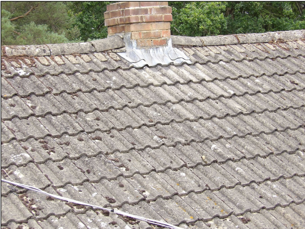
Figure 6. Example of flush lead flashing. 2 Ardwell Close, Crowthorne. 15.07.25
