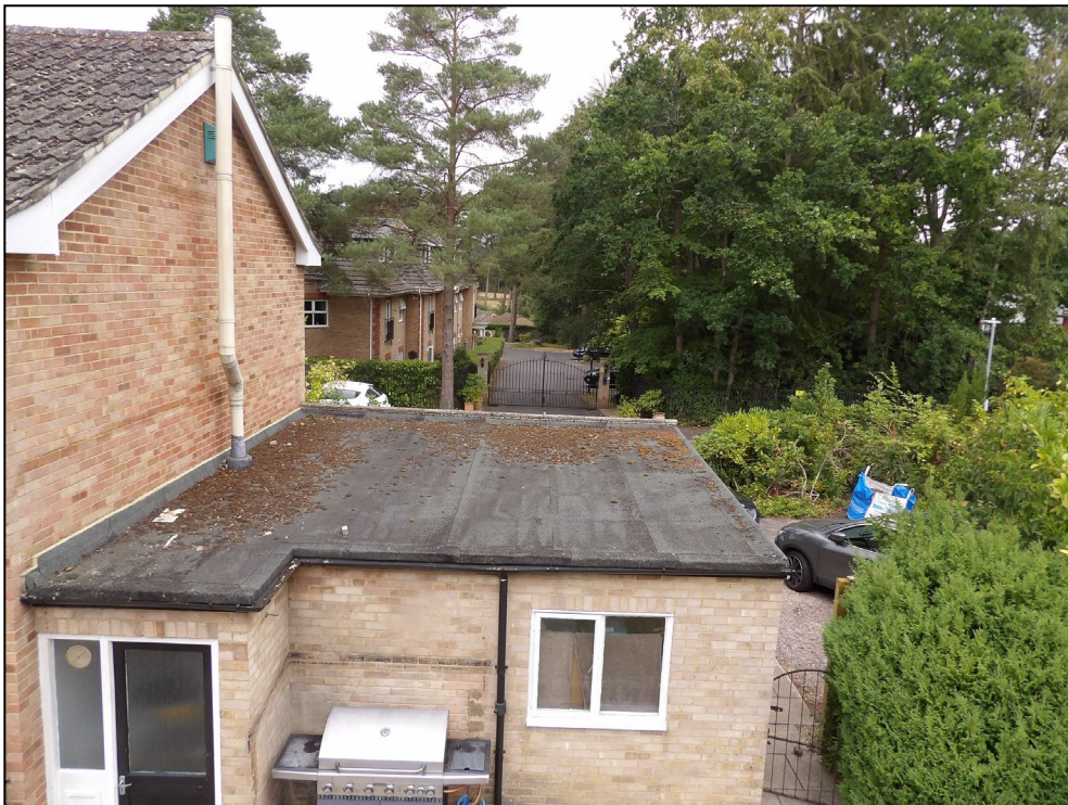
Figure 12. Bitumen covering the garage roof. 2 Ardwell Close, Crowthorne. 15.07.25
