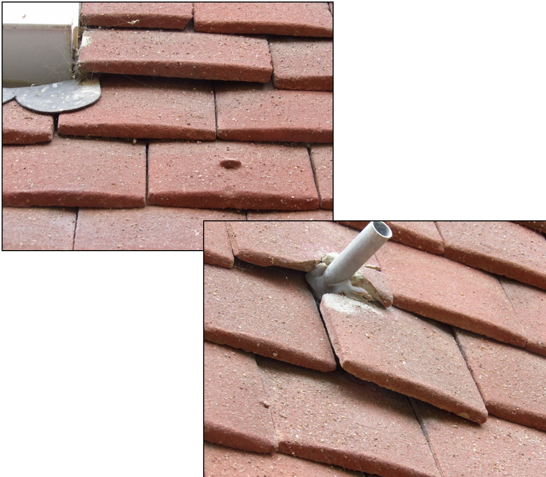
Figure 8. Example of gaps in hanging tiles. 2 Ardwell Close, Crowthorne. 15.07.25
