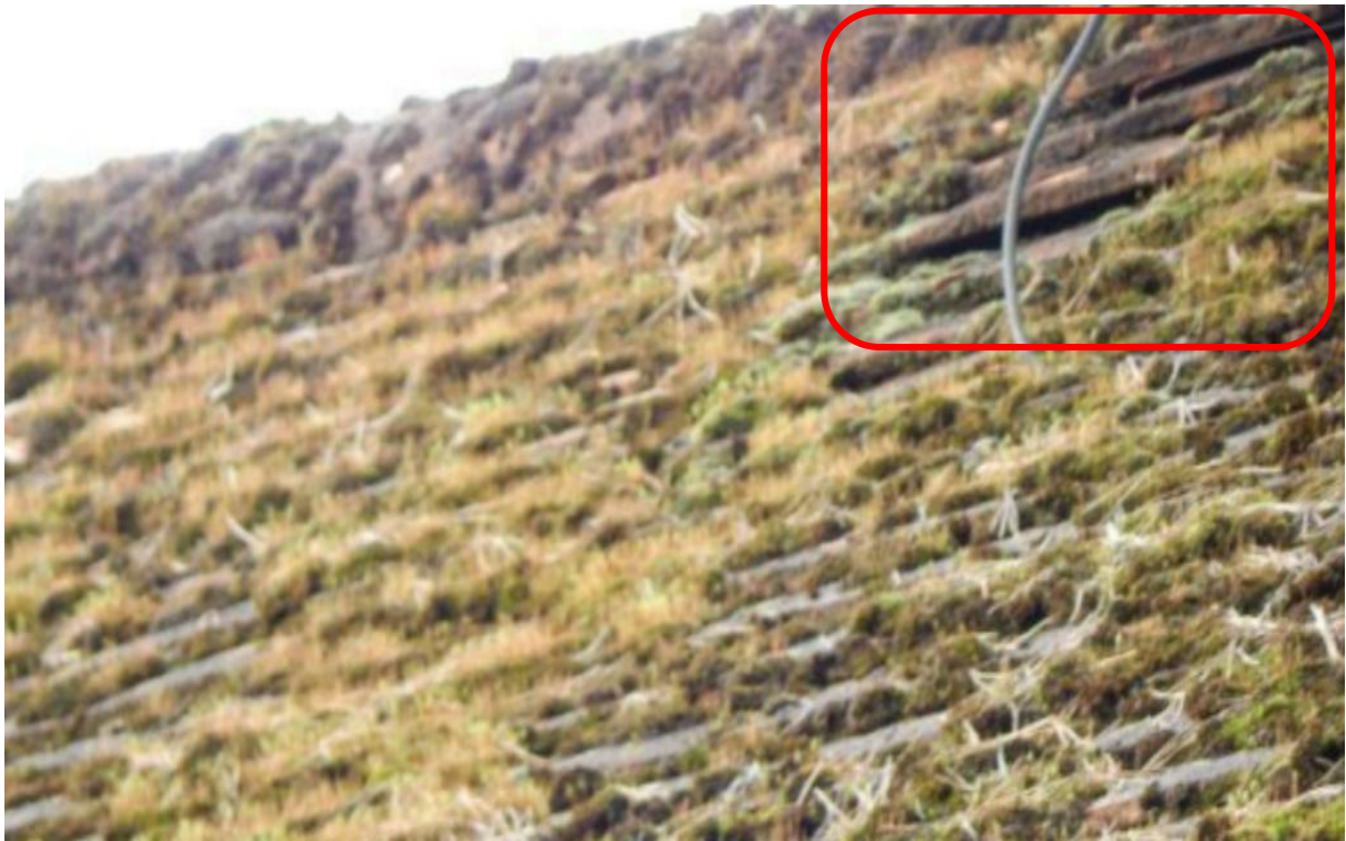
Image 3 – As per image one, raised tiles below the ridge areas of the South facing roof coverings which look to provide likely shelter/access opportunities for bats
