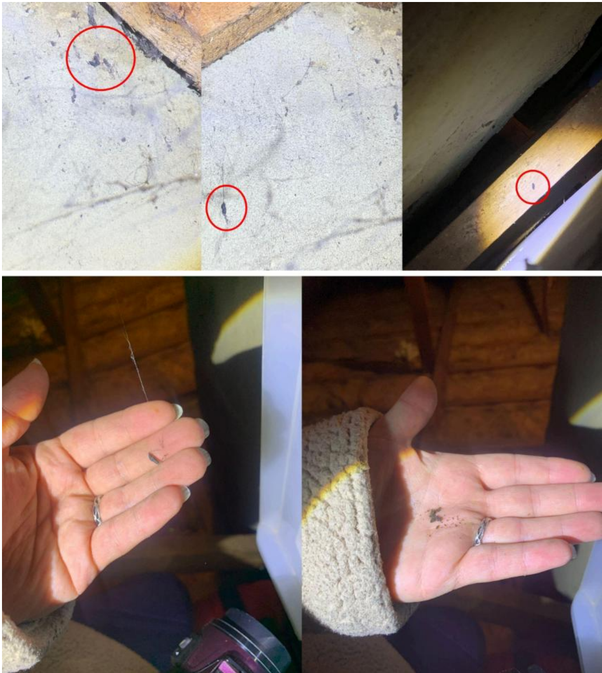
Image 9 – Evidence of as small amount of bat droppings (>5) attached to the inner chimney and floor areas surrounding the chimney confirming activity from roosting within
