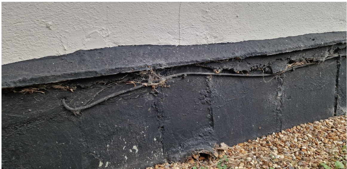
Detail of existing BT cable entry in to property
