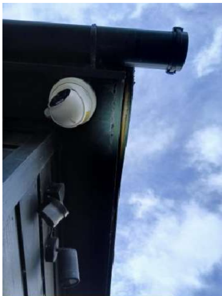
Plate 7: Small crevice near northern corner of the building
