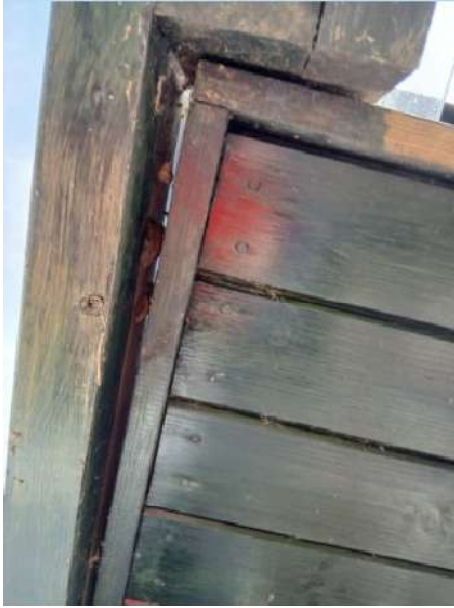
Plate 9: Small crevice on south-west elevation between sections of roof over the decking area
