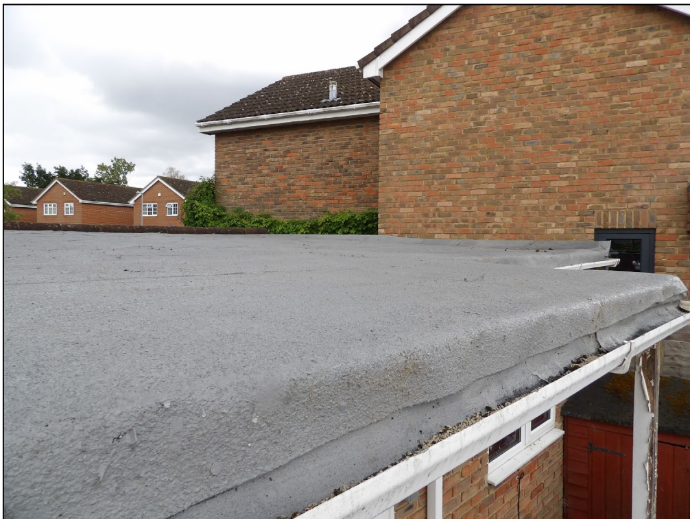
Figure 9. Example close fitted bitumen felt on spare room/garage/utility. 14 Eastbury Park, Winnersh. 22.07.25
