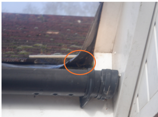
Photograph 9. Gap at garage/porch join ( TN3 ).
