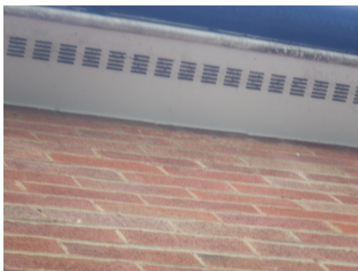
Photograph 15. Soffits tight to brickwork.
