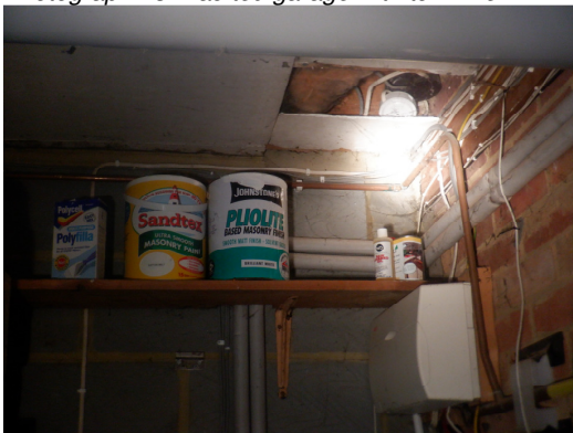
Photograph 25. Gap in boarded ceiling sheets.
