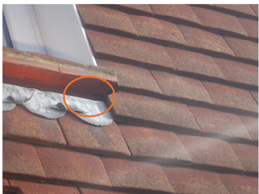
Photograph 12. Gap under windowsill leading behind hanging tiles ( TN4 ).
