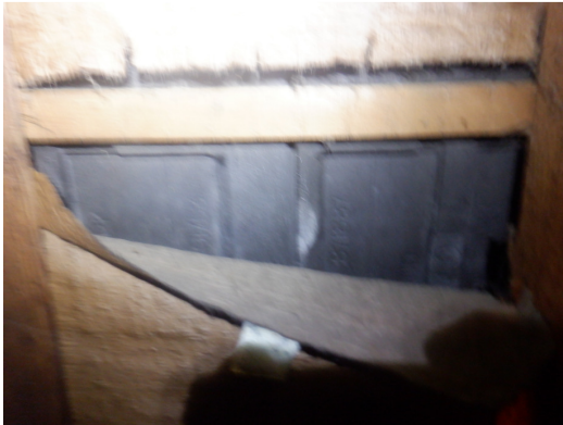
Photograph 17. Flat roof tiles visible in paper liner tears/gaps (TN7).
