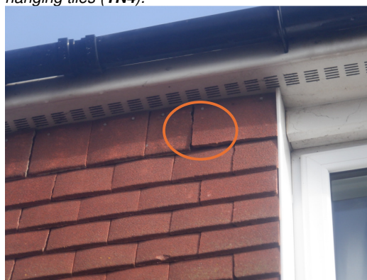
Photograph 13. Gap under top course of hanging tiles ( TN4 ).
