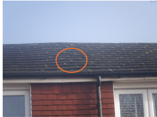
Photograph 4. Raised curve in roof tiles at extension line.
