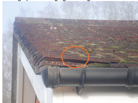
Photograph 8. Slightly lifted garage verge tile ( TN2 ).
