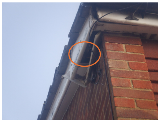
Photograph 16. Broken soffit on northern elevation (TN6).
