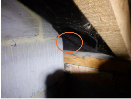
Photograph 22. Gap at northern blockwork gable edge, daylight visible (TN14).
