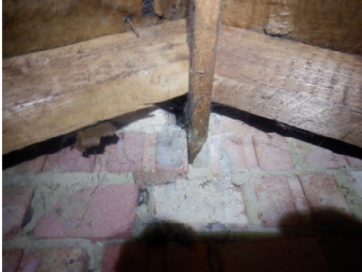
Photograph 19. Cobwebbed ridge beam (TN9).
