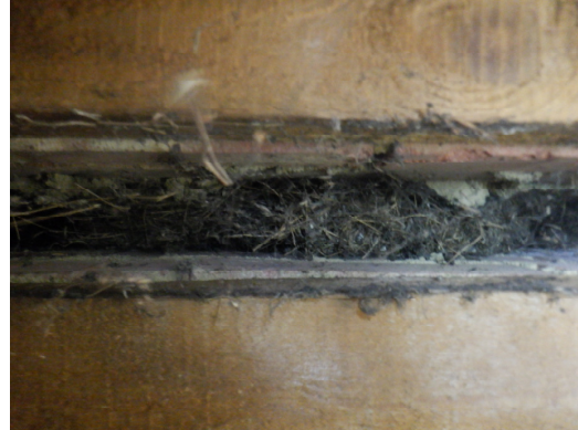
Photograph 20. Bird nesting material in old external cavity wall (TN10).
