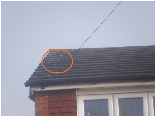
Photograph 3. Lifted tile on front elevation ( TN1 ).
