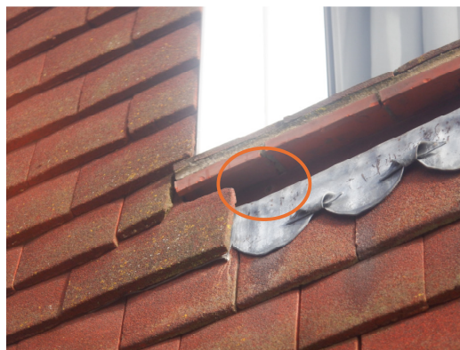
Photograph 11. Gap under windowsill leading behind hanging tiles ( TN4 ).
