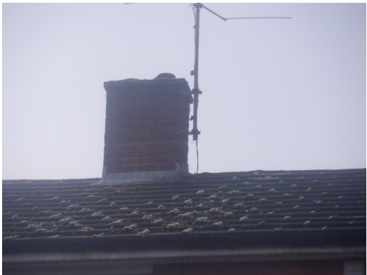
Photograph 5. Moss on rear elevation tiles.
