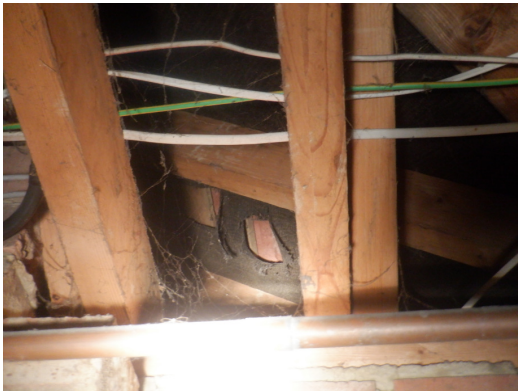
Photograph 23. Vaulted garage with torn liner.
