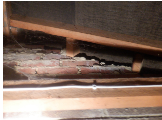
Photograph 24. Gaps at edge of gable brickwork.
