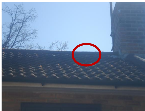
Photograph 6. Crumbling verge mortar (rear elevation).
