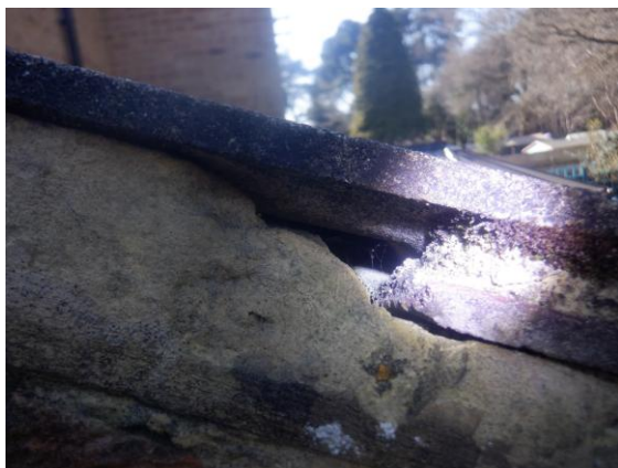
Photograph 5. Gap of limited extent behind crumbling verge mortar (east elevation).
