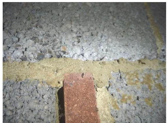
Photograph 12. Medium-sized bat droppings stuck to gable wall in side extension.
