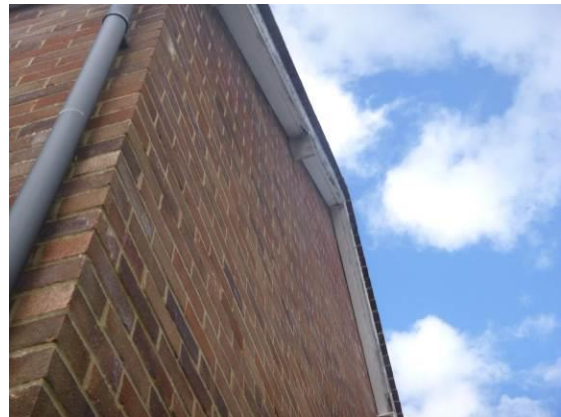
Photograph 5. Gaps behind gable soffits on extension (side elevation).
