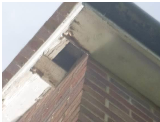
Photograph 6. Hole in soffit box at extension end (side elevation).
