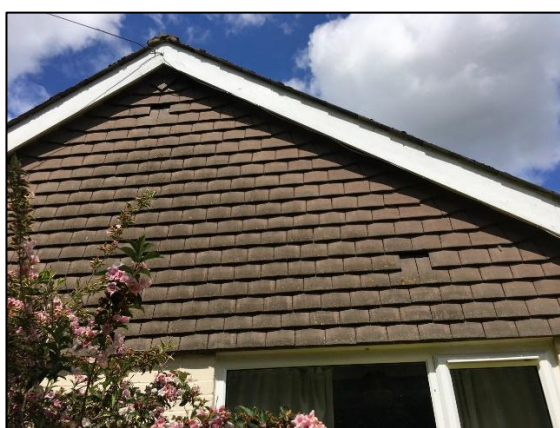
Photo 37 Slipped tiles (B1)
