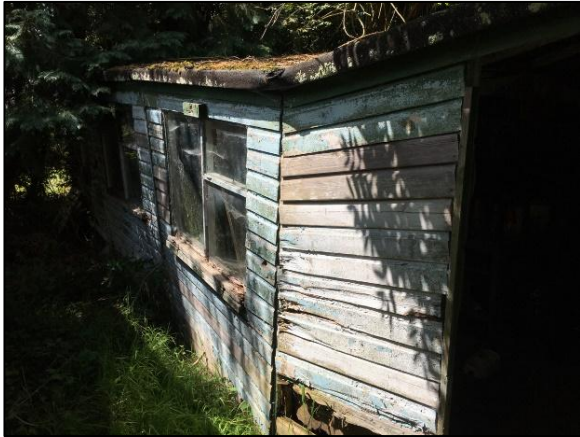
Photo 57 Dilapidated structure (B5)
