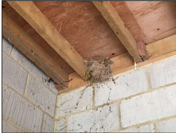
Photo 67 One of ten house martin nests within B3
