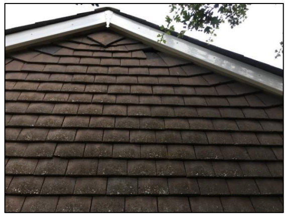
Photo 42 Missing wall tile (B2)
