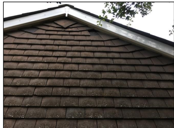
Photo 66 Bird nesting behind slipped tile
