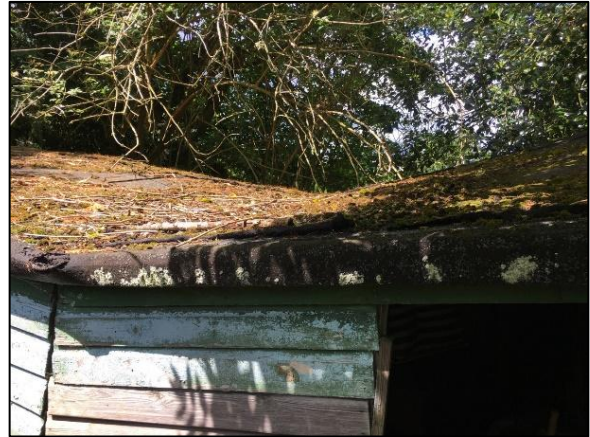
Photo 58 Dilapidated structure (B5)
