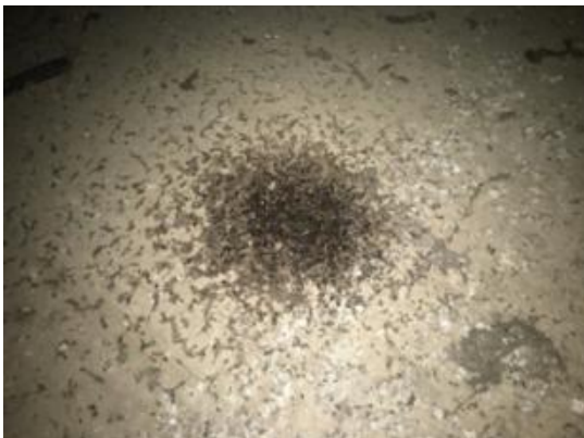
Photo 72 Building B3 – clustered bat droppings
