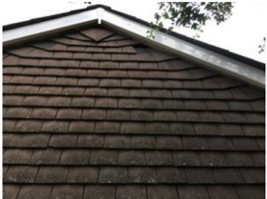
Photo 66 Building B2 – missing tile
