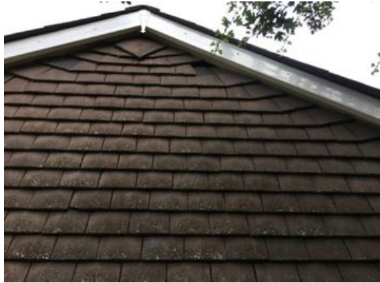
Photo 95 Bird nest behind missing tile on B2
