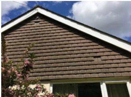
Photo 64 Building B1 – missing tiles
