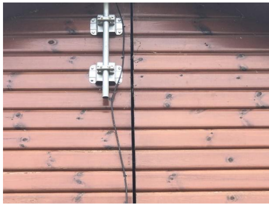
Photo 83 Building B8 – split in panelling
