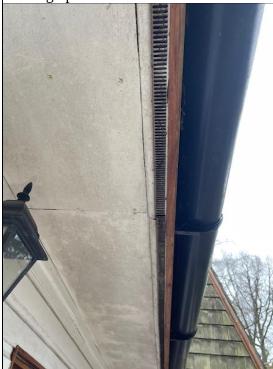
Photograph 19: No gaps around guttering or soffits.
