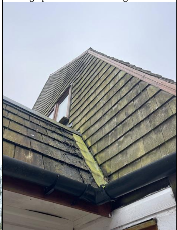
Photograph 20: No gaps around hanging tiles.
