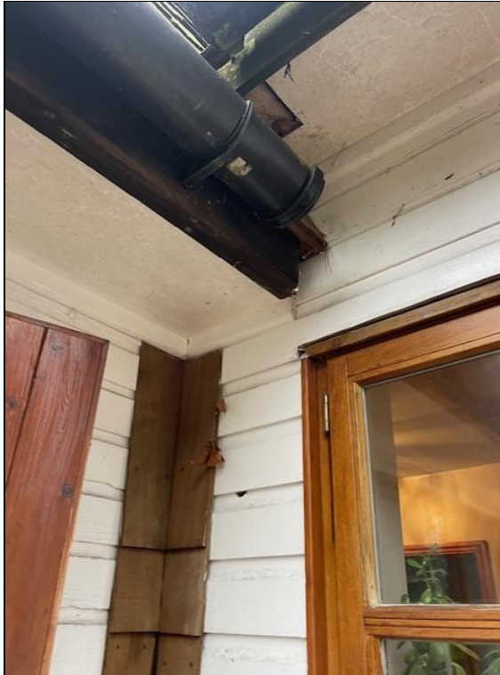
Photograph 21: Gaps around porch.
