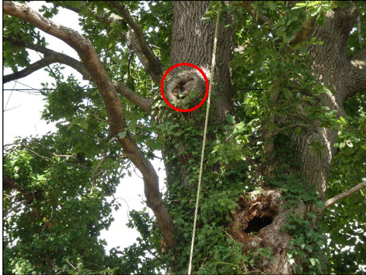
Figure 2. Cavity on northern stem. Oak at 9 & 10 Bradely Drive 26.08.2025
