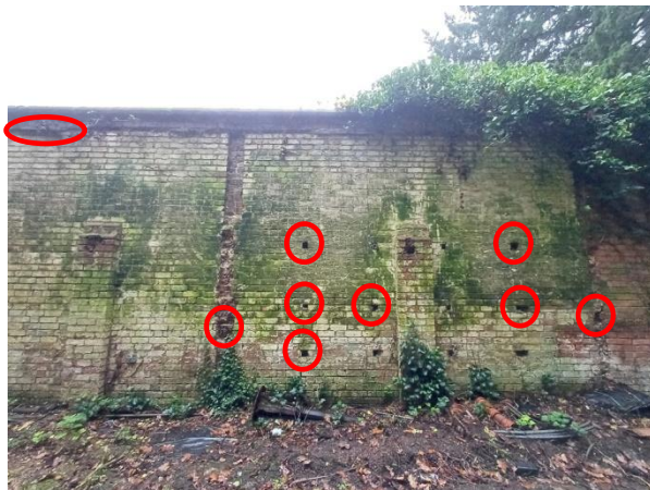
Plate 11: PRF's on exterior north elevation of northern wall (red circles)
