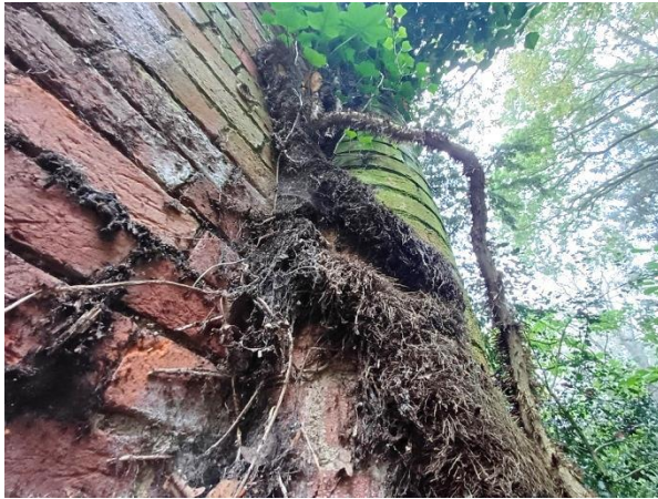
Plate 13: Thick-stemmed ivy on exterior north elevation of northern wall
