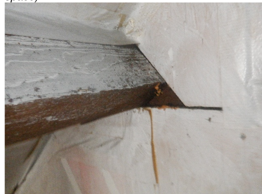
Photograph 24. Gaps around edges of timbers in eave space (front elevation)
