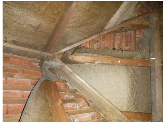
Photograph 19. Large tears in the roofing felt (First roof void).
