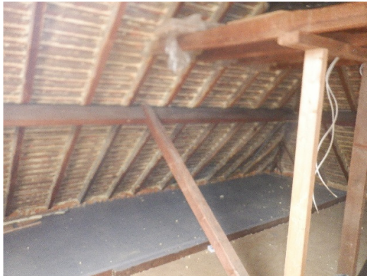
Photograph 14. Void of cut & pitch construction (First roof void).
