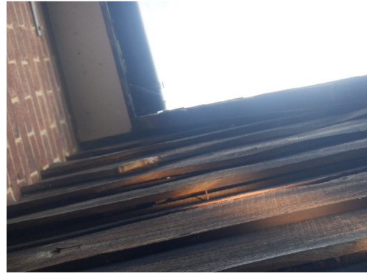
Photograph 13. Gaps under the waney edge boards (rear elevation).
