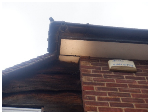
Photograph 6. Gap of limited extent between sheets of timber at the soffit (rear elevation).
