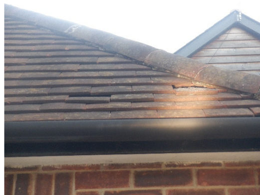
Photograph 8. Slipped roof tiles on the single storey hipped roof (Rear elevation)
