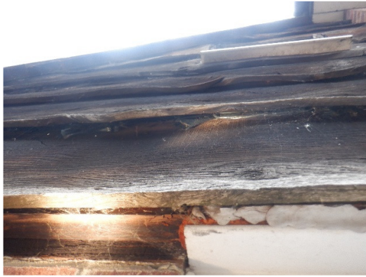
Photograph 12. Gaps under the waney edge boards (front elevation).
