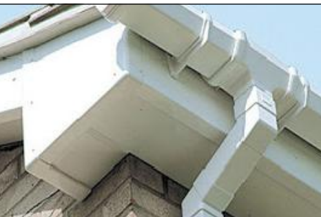
WHITE UPVC FASCIAS AND GUTTERS
