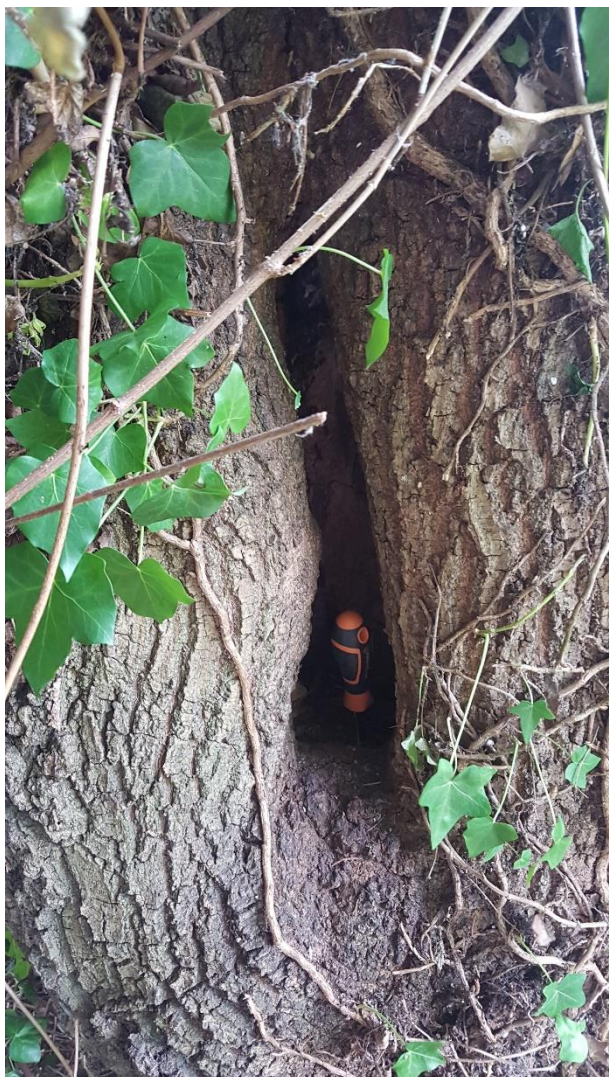
Photo 1 – Cavity on south side with metal probe.
