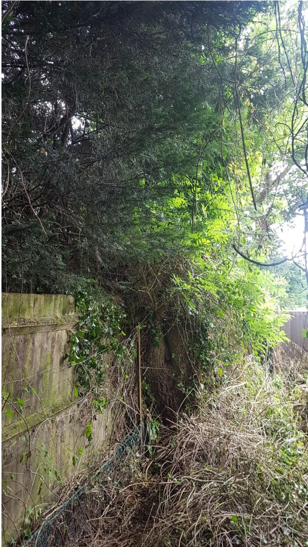
Photo 3 – Base of tree growing adjacent to boundary
