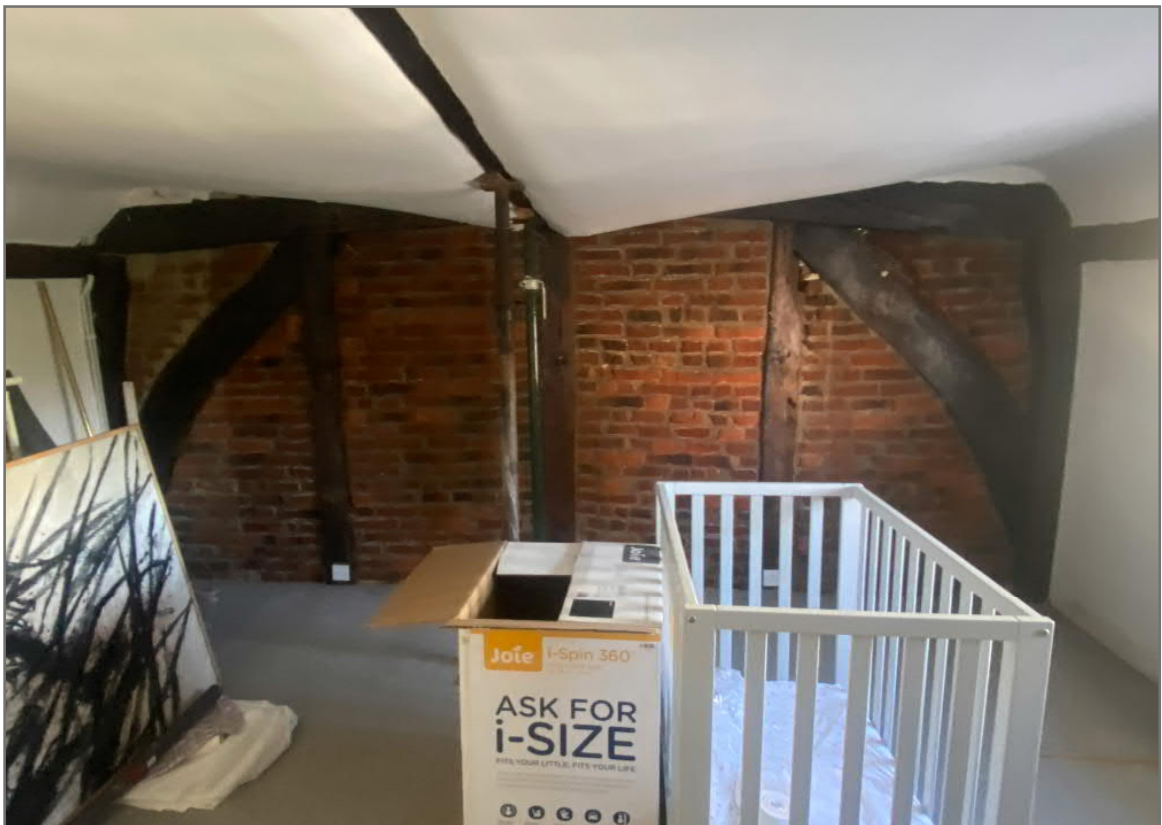
Image 15: Exposed internal timber construction to the First Floor West gable (typical): proposal to remove all modern impervious paints and varnish to all historic timbers using soda blasting
