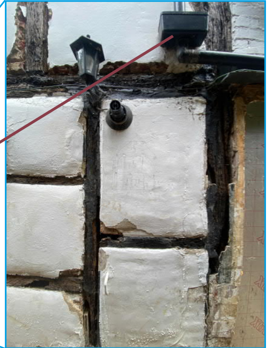
Image 05b: Detail of existing boiler flue
