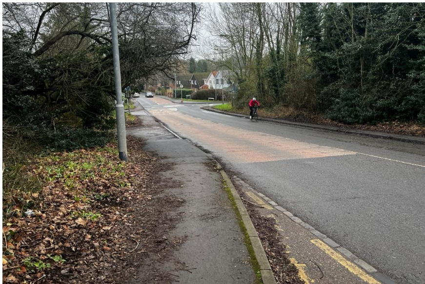
Photograph 6: Condition of Barkham Road
