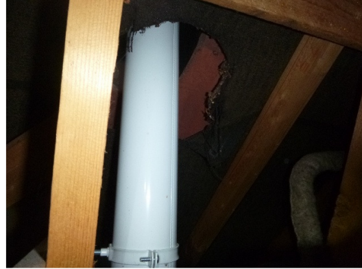
Photograph 12. Gap in felt around flue pipe.
