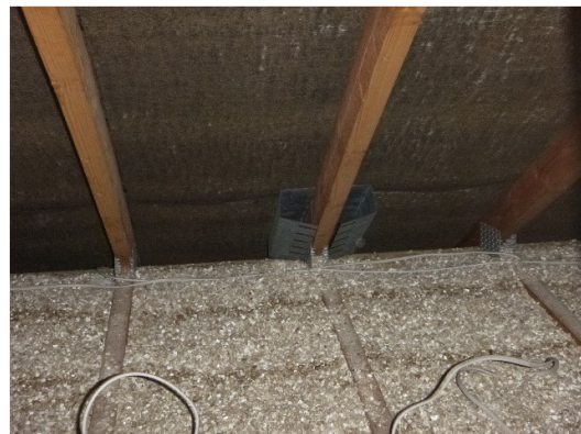
Photograph 16. Open eaves and floor with vermiculite chippings.
