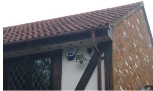
Photograph 9. Verges fully mortared at eastern gable.
