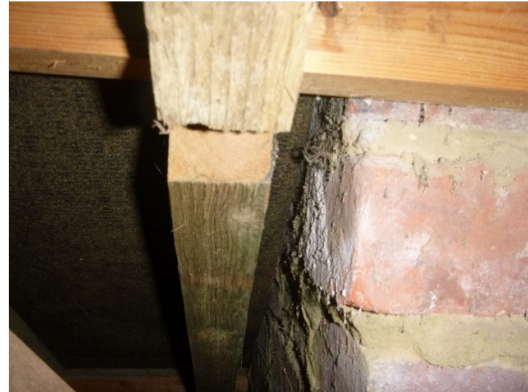
Photograph 14. Felt tight around chimney.
