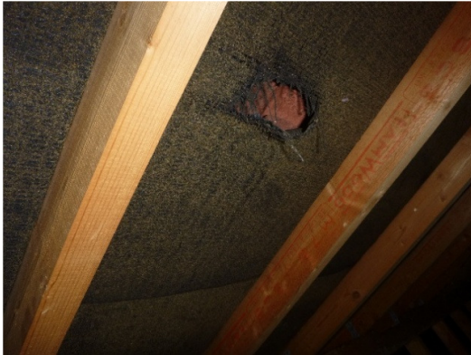
Photograph 13. Small tear in roofing felt.
