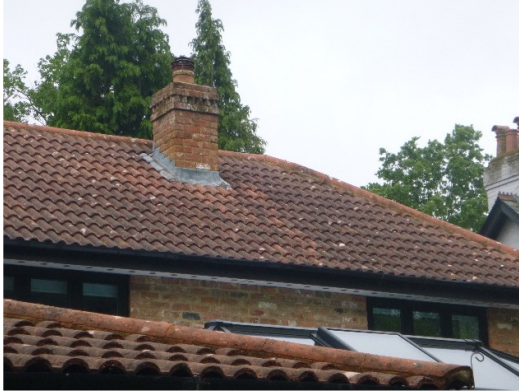
Photograph 3. Tight interlocking tiles (rear elevation).
