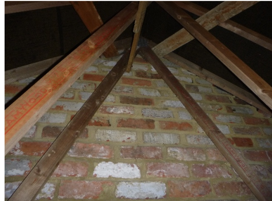
Photograph 20. Brick work gable end of the garage tight to the timbers and felt.
