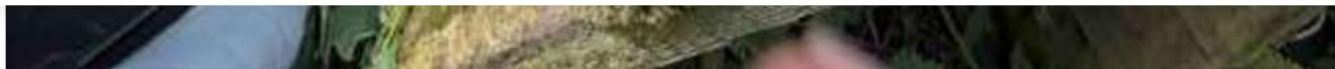
Figure 9: North side of T1 base showing extensive historic wound
