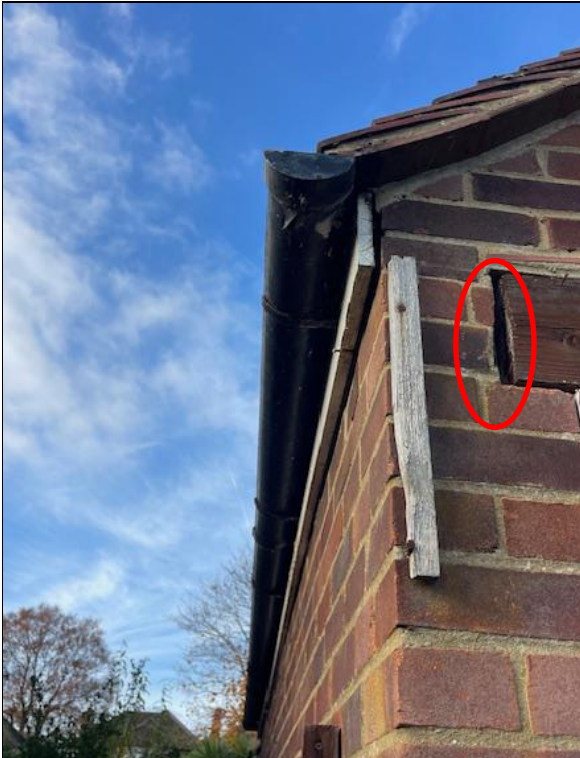
Photograph 25: Gap between the wood and the bricks on the garage- fully inspected.
