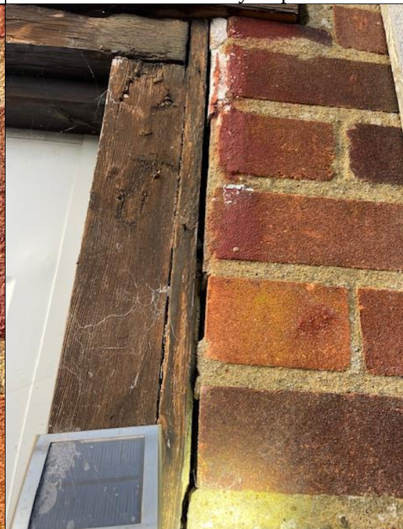
Photograph 24: Gap between the wooden frame and the mortar on the garage.
