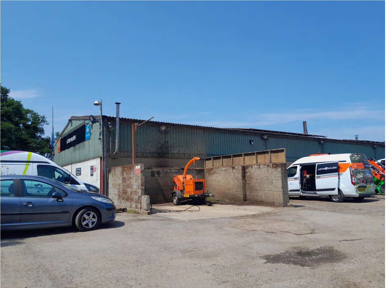
View of vehicle washing bay at the southern end of the concrete brick and corrugated metal vehicle maintenance workshops in the centre of the site. Surface covering is poured concrete, cracking is visible.
