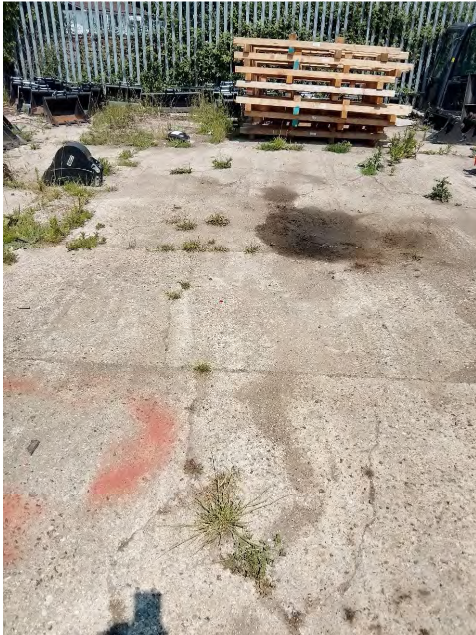
Photograph of external storage area with concrete slab surface covering with discoloration and cracking visible in the centre of the site.
