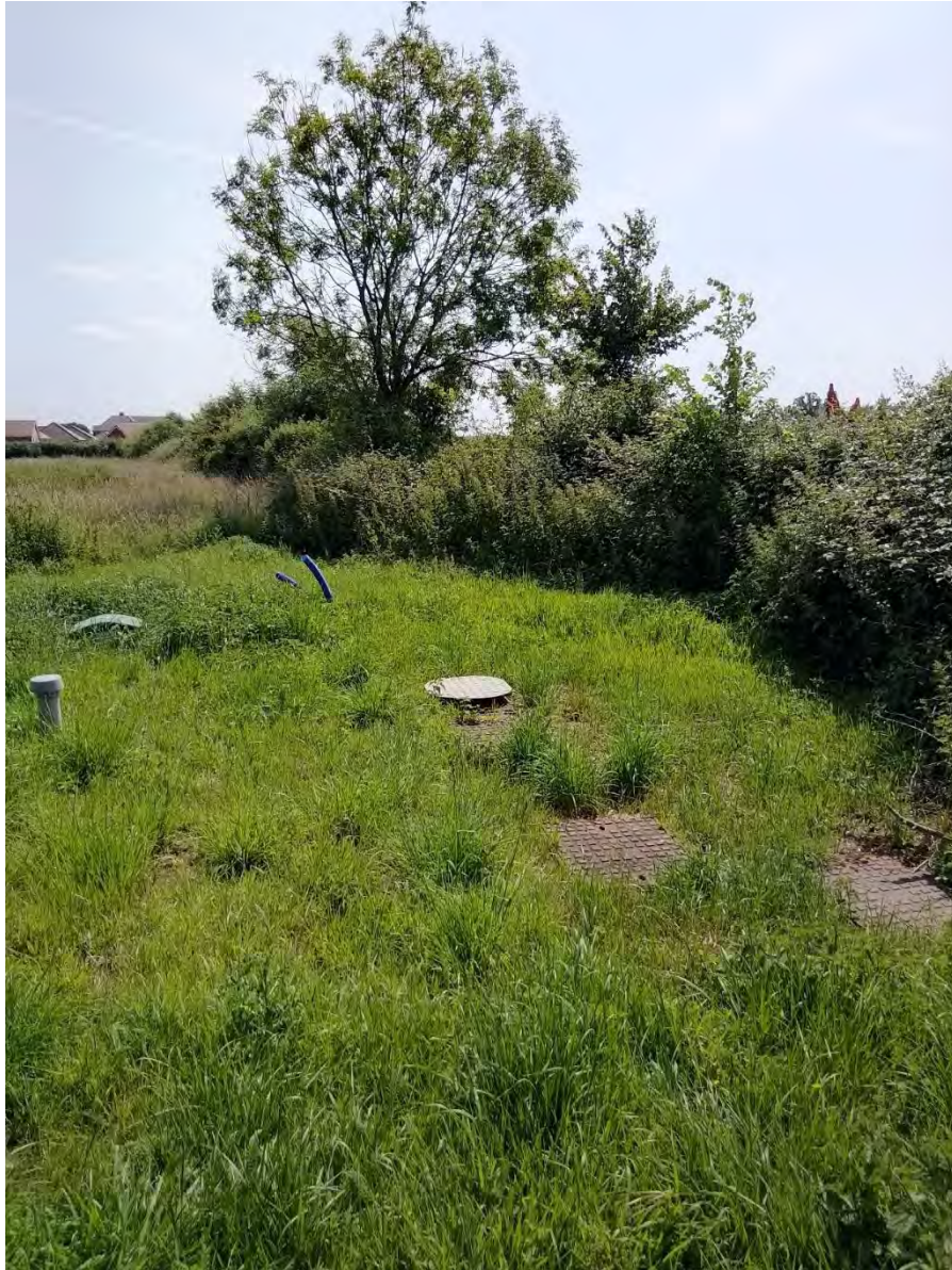
View of existing drainage infrastructure with septic tank ventilation and inspection covers looking east. The image has been taken beyond the northern boundary, comprised of hedgerows with mature shrubs and scattered trees, in the field to the north of the site
