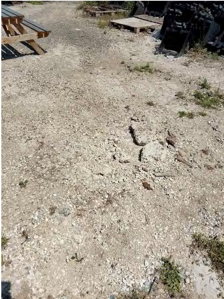
Broken concrete slab in external storage area in the western area of the site.
