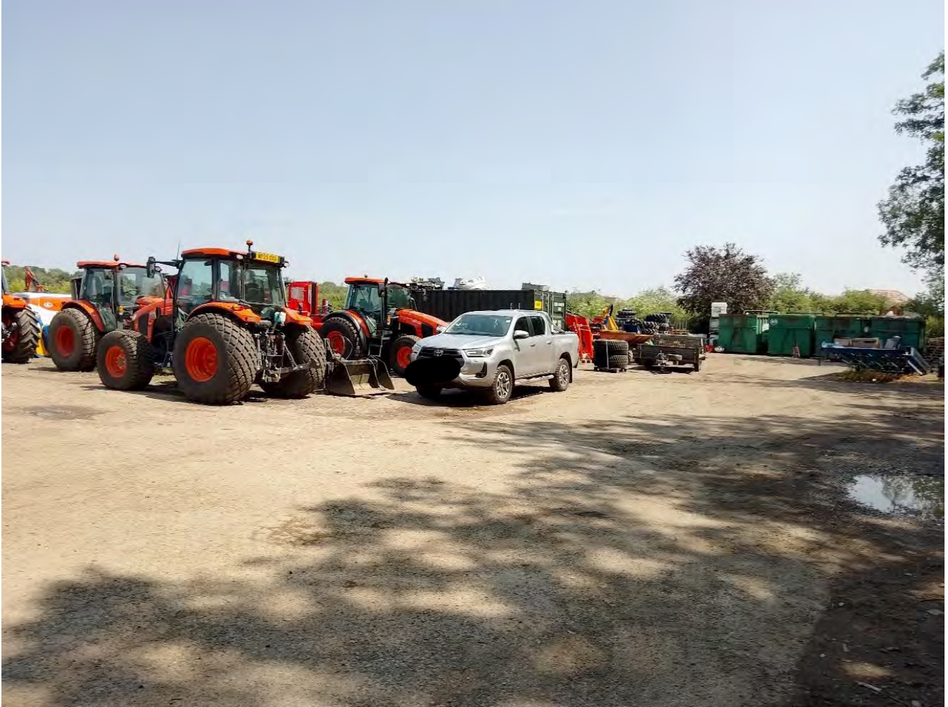
View of the southern vehicle and machinery storage yard in the centre of the site looking northeast. Surface covering is poured concrete, cracking is visible.
