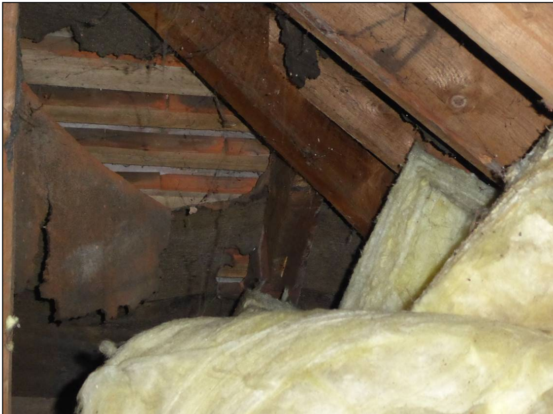
Figure 15. Ripped bitumen lining. 220 London Road, Wokingham, 05.07.24
