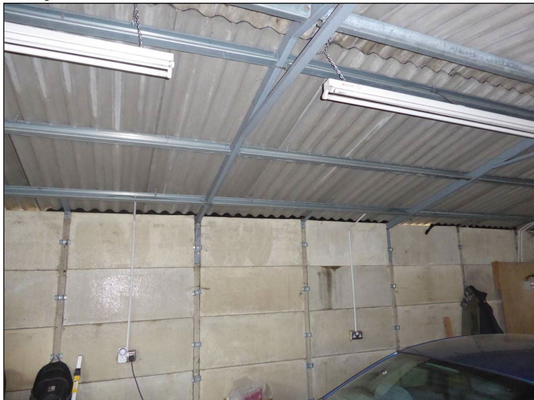
Figure 17. Exposed fibre cement sheeting roof of garage. 220 London Road, Wokingham, 05.07.24
