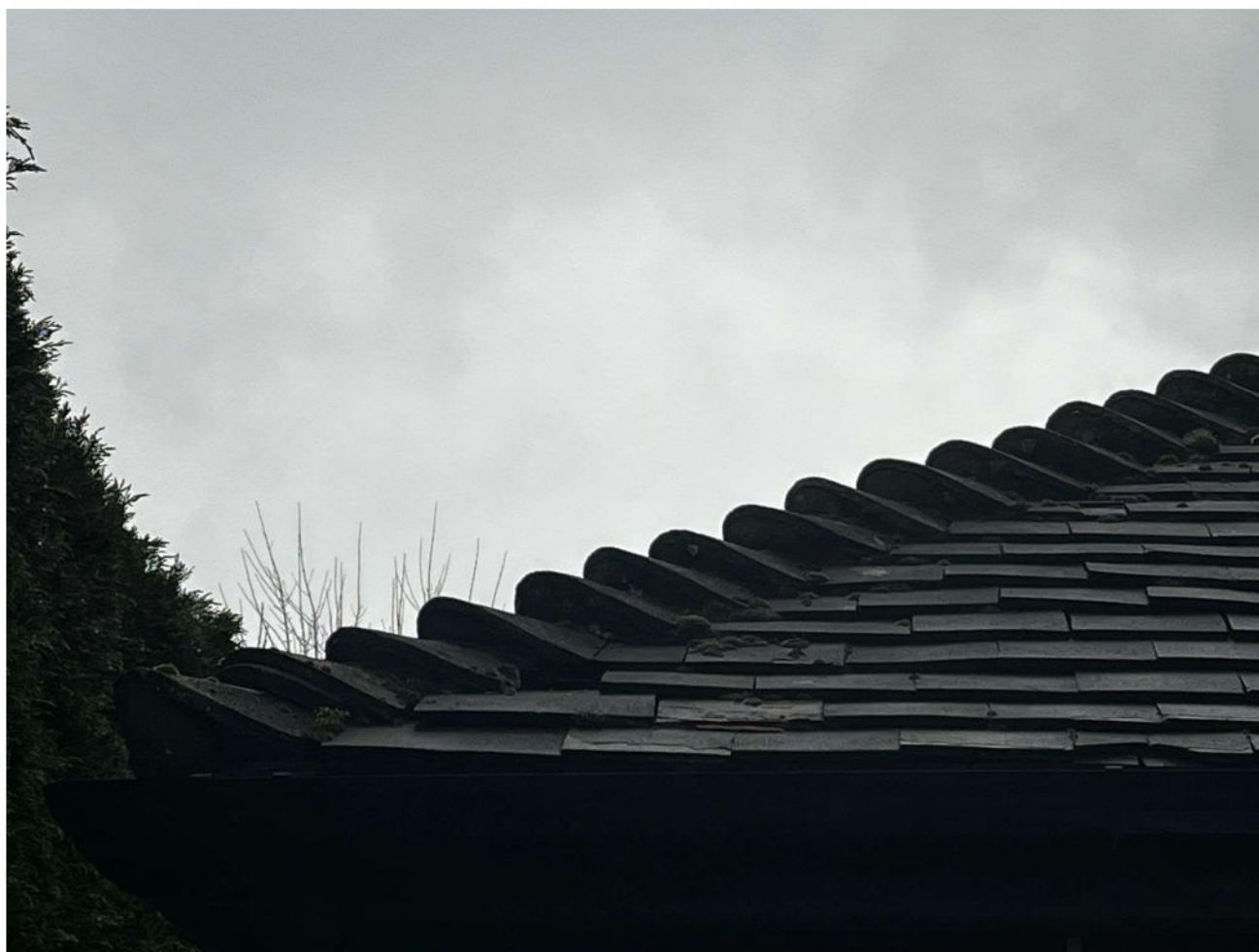
Image 3 – Lifted roof tiles – not a big enough gap to be a potential roosting feature
