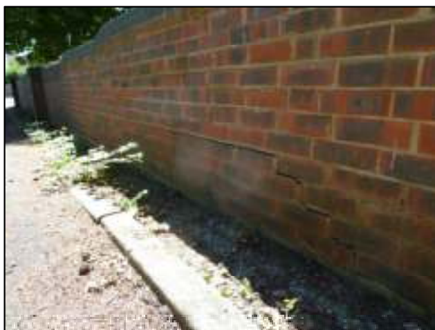
Photograph 1: Cracking at base of wall, South Lodge. 30.6.2015.
