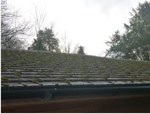
Photograph 6. Flat and mossy plain roof tiles (north elevation).
