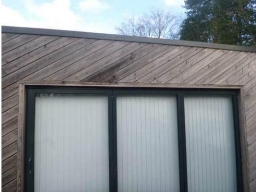
Photograph 14. Tight timber cladding on detached office (eastern elevation).
