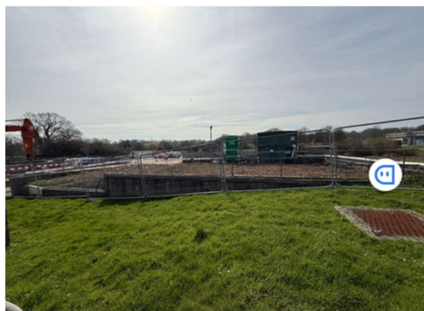
Photograph 3 – Sludge Drying Beds
