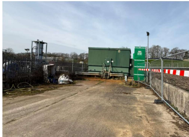
Photograph 5– Chemical Dosing Area
