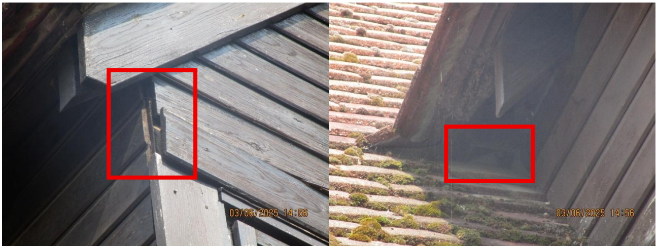
Photo 9 – Gap in brickwork, and Photo 10 - Gaps between bargeboard and wall
