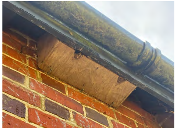
TN2 - Potential bat box under soffit on rear elevation of B1
