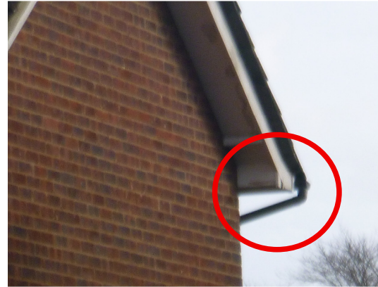
Photograph 11. Damage to soffit at the western end of the roof.
