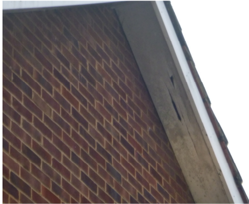
Photograph 10. Damage to timber soffits and small gaps between soffit and brickwork and intact uPVC fascias (eastern elevation).
