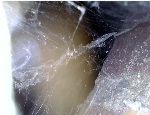
Photograph 14. Cobwebbed gap checked with an endoscope beneath the verge on the eastern elevation.
