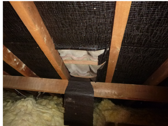
Photograph 18. Large tear in bitumen felting to the south of the loft hatch (roof void).
