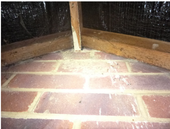
Photograph 21. Small gap between timber rafters and previous external wall with bird droppings visible (loft void).
