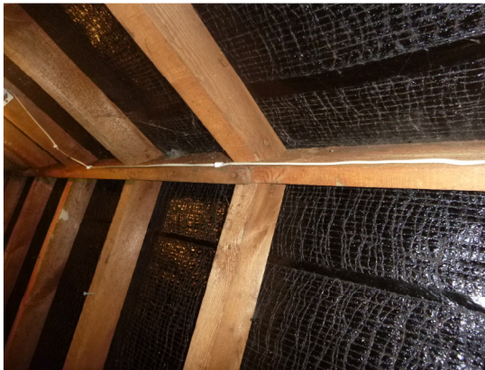
Photograph 17. Mostly intact bitumen felting across roof void (roof void).
