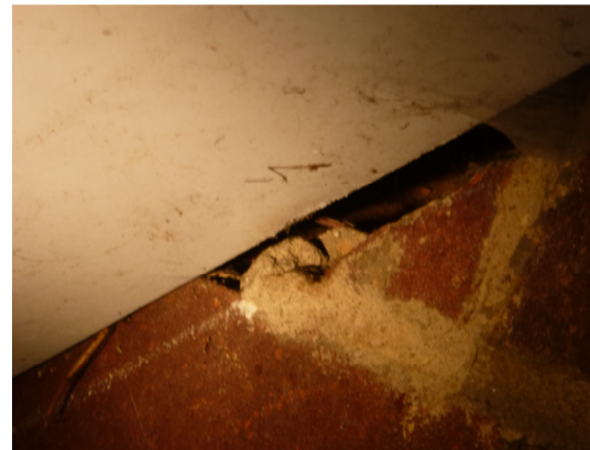
Photograph 13. Gap in brickwork beneath verge on the eastern elevation of the sloping roof (eastern elevation).
