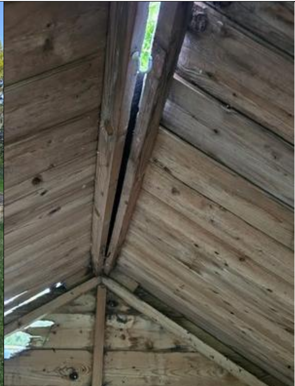
Photograph 22: Large gaps in shed C.
