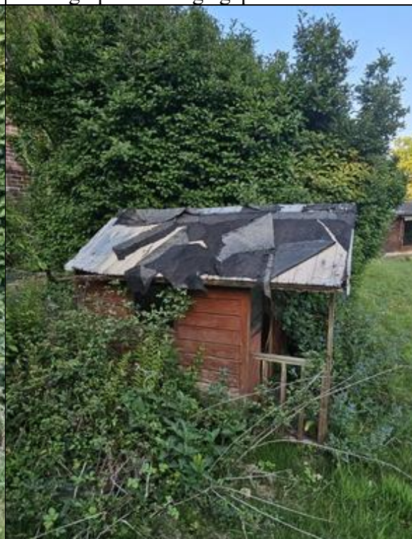
Photograph 24: Derelict shed C.
