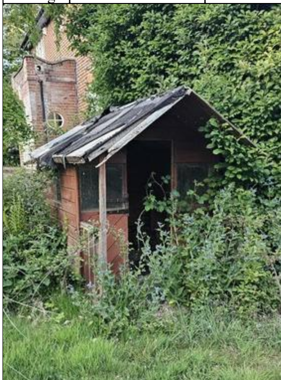
Photograph 23: Derelict shed C.
