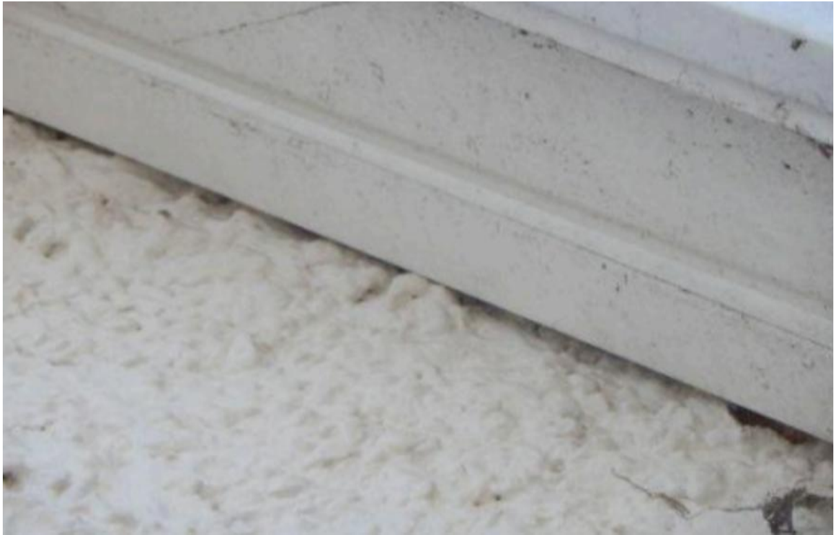
Image 5 – Minor gaps between the eaves and render coverings which may provide access opportunities for bats within
