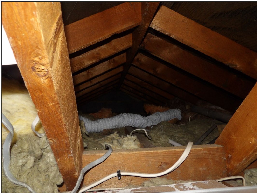
Figure 13. Internal view of remaining loft space and torn bitumen felt. 30 Byron Road, Twyford. 20.01.26
