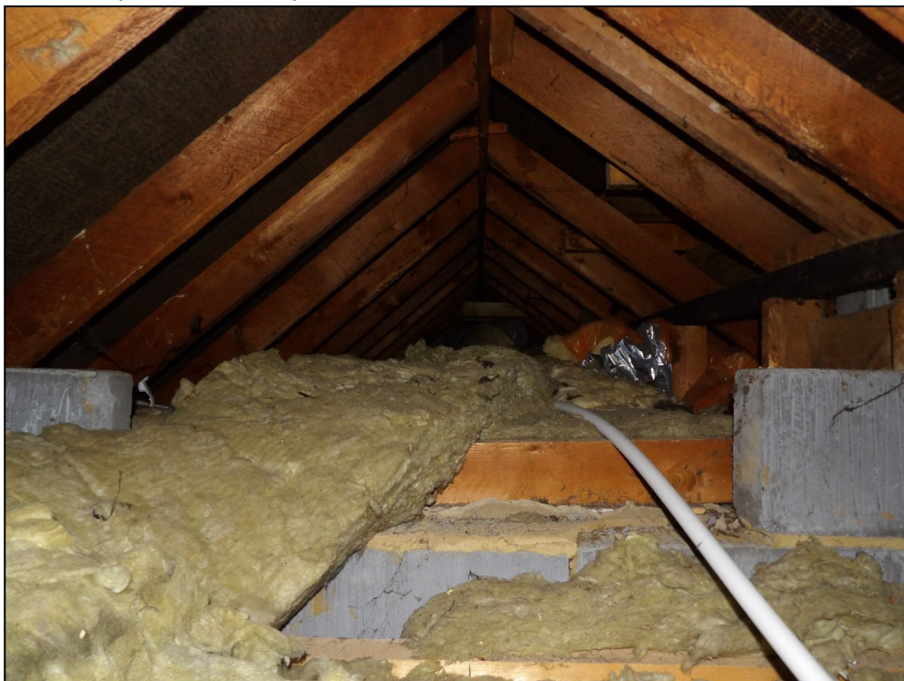
Figure 15. Internal view of loft space above attached annex and bitumen felt lining to tiles. 30 Byron Road, Twyford. 20.01.26
