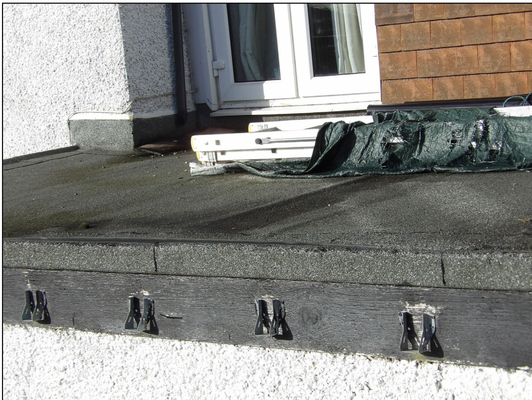
Figure 12. Example sealed fascias on rear extension. 30 Byron Road, Twyford. 20.01.26
