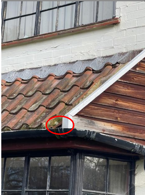
Photograph 11: Gaps around roof tiles.
