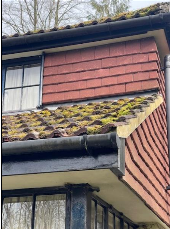
Photograph 9: Hanging wall tiles.
