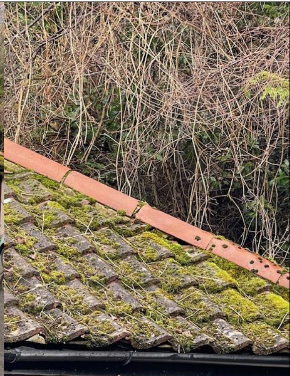
Photograph 2: Gaps under roof tiles.
