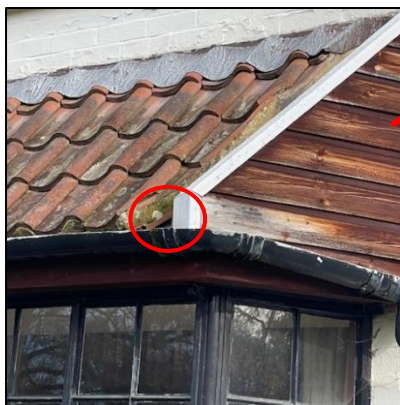
Raised roof tiles.
