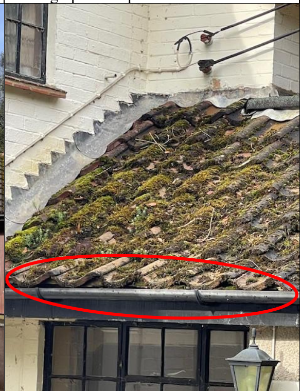
Photograph 4: Gaps under roof tiles.
