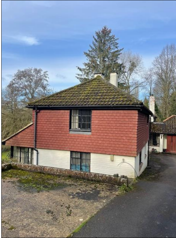
Photograph 7: Hanging wall tiles on the side elevation.
