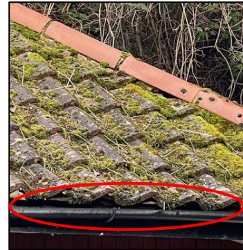
Gaps under roof tiles on garage.
