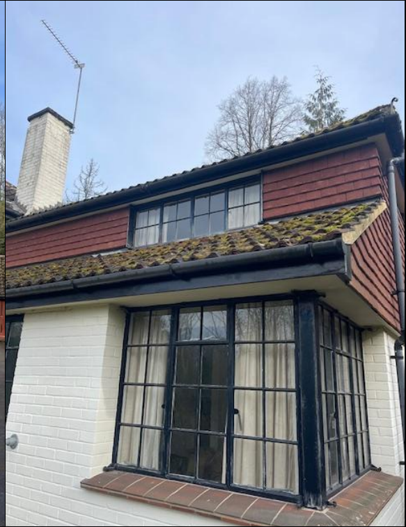
Photograph 8: Hanging wall tiles.
