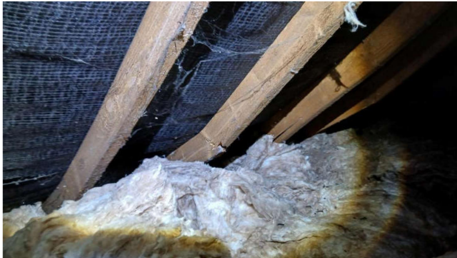
Image 4 – View from within loft space of cellar showing deflected and failed modern rafters.
