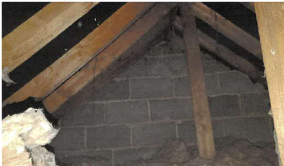
Image 5 – View from within loft space of cellar showing deflected modern rafters.
